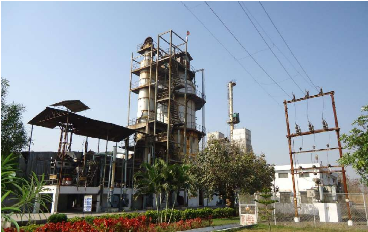
Incinerator Capacity : 5.5 mkcal/hour
